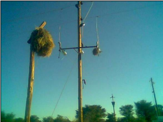
Dummy pole on Farm Eldorado (pump) on Kalkpan reticulation line, 153km from Aranos (see dummy on left, and smaller nest on the cross-arm structure)
