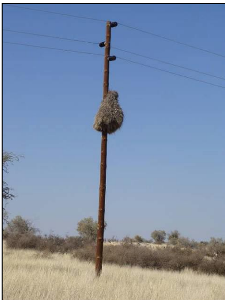
Basket (made out of old conductor wire) on Kalkpan HLPCD (horizontal line post compact delta) reticulation line, Farm Dai Gratia.
