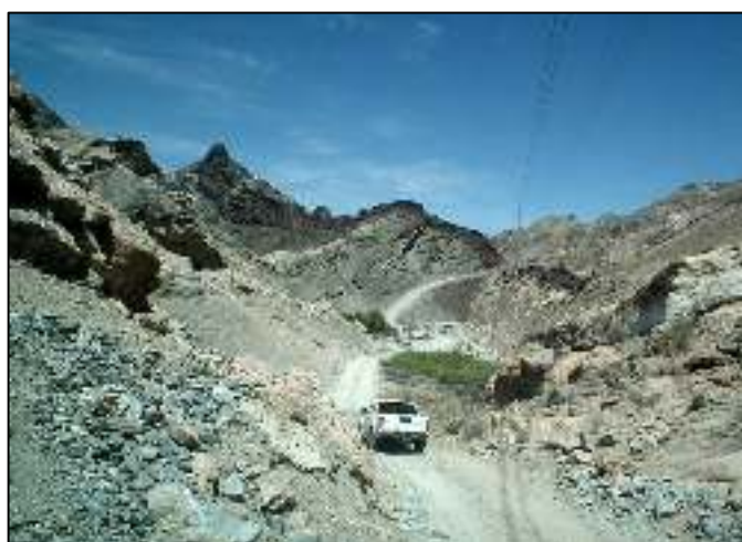
The new Lithops-Husab power line runs through some extremely rugged terrain (photos Ann Scott)
