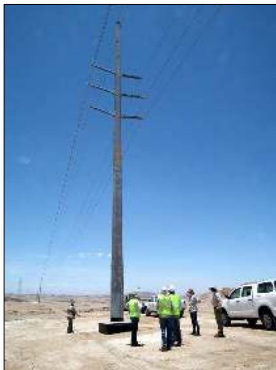
The new Lithops-Husab power line uses a steel-type monopole about 25 m high; the (horizontal) insulators are 1.5 m long
